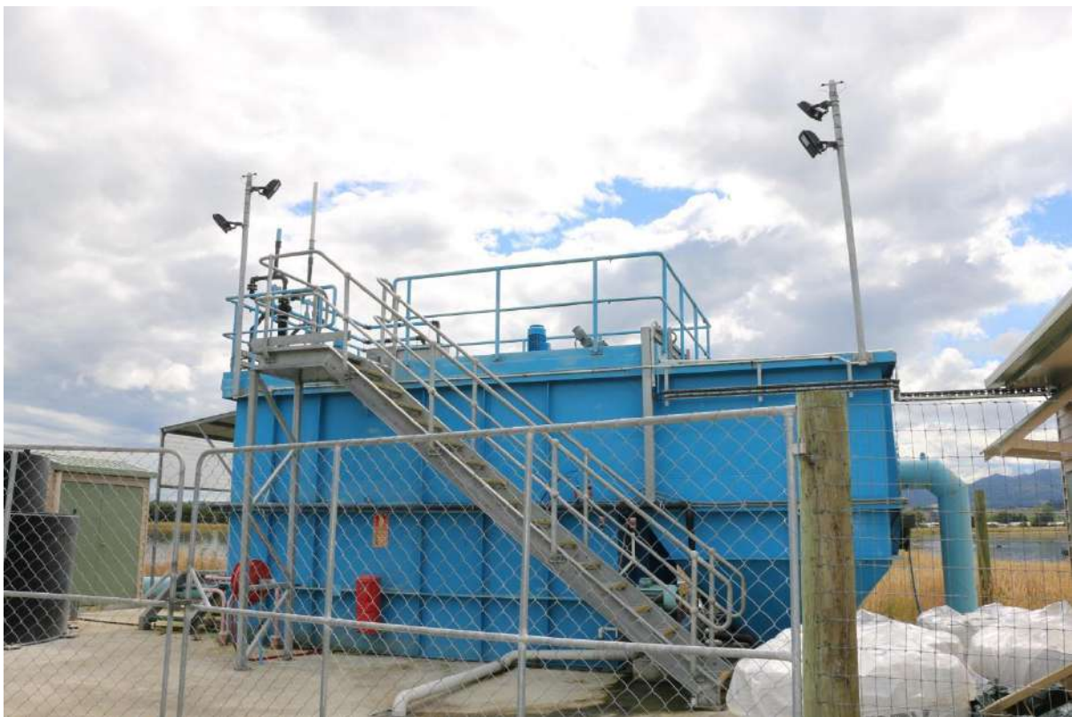
Image 14.1: Gore's Actiflo plant (a chemical treatment process to reduce phosphorous and suspended solids)
