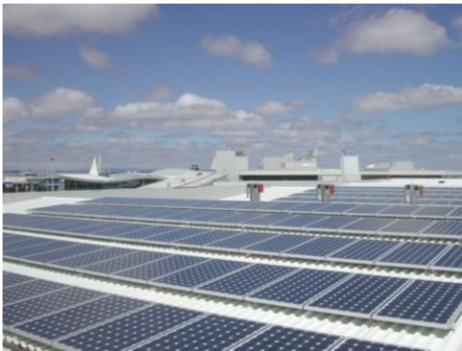
Figure 7.1: Auckland international airport stage 1 grid tie installation, 51 kWp (Sharp modules installed by Reid Technology)
